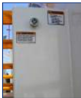
Hydraulic oil tank sight gauge and WARNING signs
