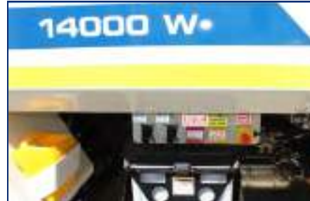
Battery isolation switch located on the control panel at the front right hand
