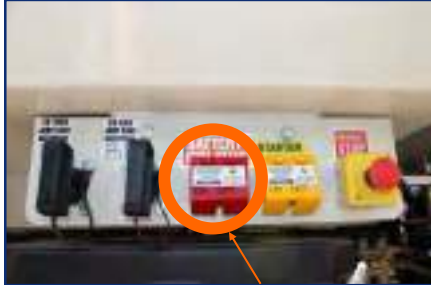
Battery Isolation Switch
