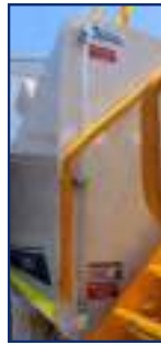
Water tank level sight gauge
